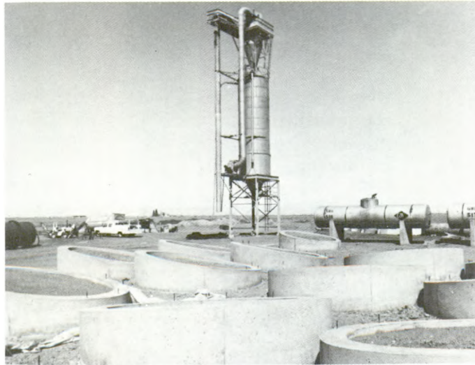
One idea for facilitating cleaning is to make tanks that have sloped bottoms for easy draining (Colorado Agro-Energy Inc. plant under construction, Monte Vista).
