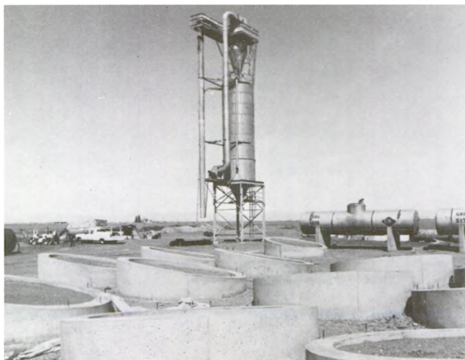
One idea for facilitating cleaning is to make tanks that have sloped bottoms for easy draining (Colorado Agro-Energy Inc. plant under construction, Monte Vista).
